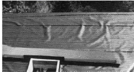
Conventional organic felts can absorb moisture, causing severe buckling and wrinkling.
