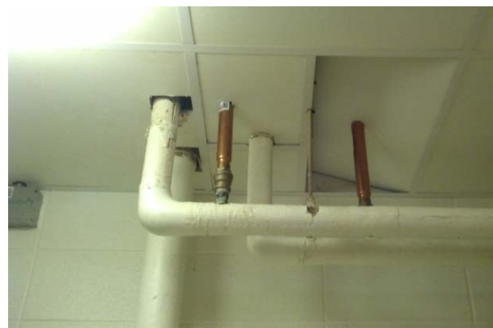
Existing Water Hammer Arrestors
