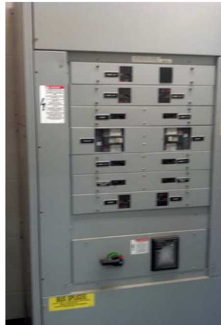
Main Electrical Switchgear
