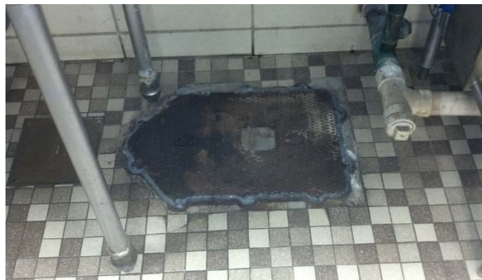
Existing Passive Grease Interceptor
