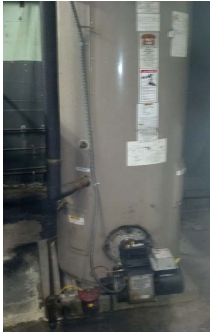
Existing Oil Fired Water Heater
