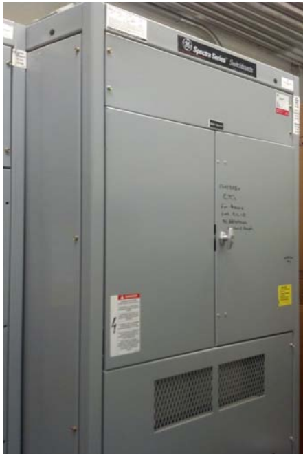
Main Electrical Switchgear
