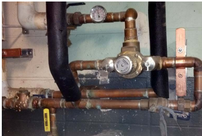
Existing Thermostatic Mixing Valve
