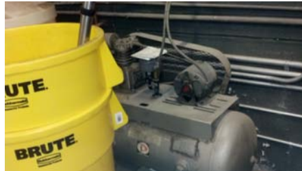
Control System Compressor
