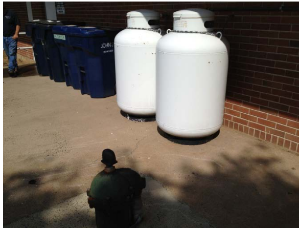
Existing propane tanks
