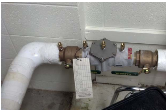
Existing Backflow Preventer
